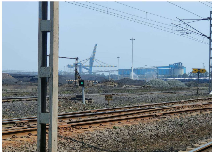
Sprinklers system for the suppression of coal dust
