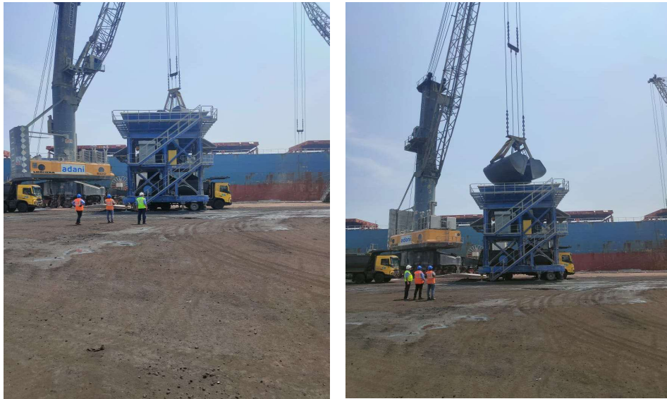
Mechanized system for loading of coal into dumpers/trucks
